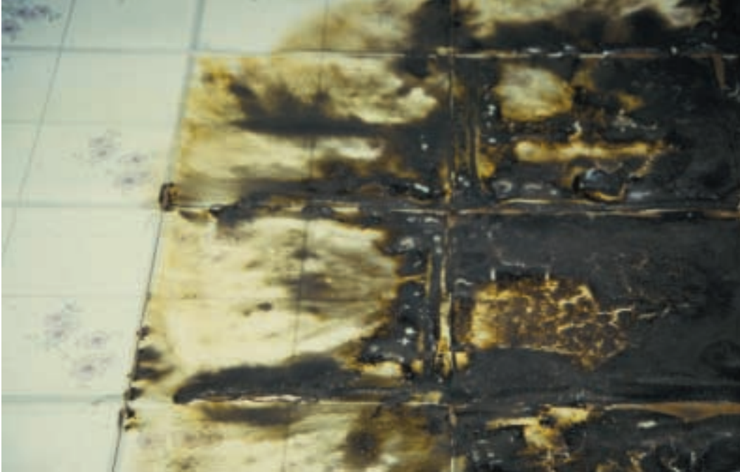
Figure 11. Closeup of gasoline spill fire pattern on vinyl floor
