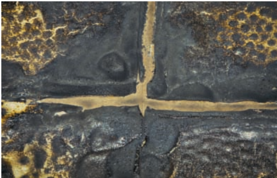
Figure 12. Closeup of gasoline spill fire burn pattern on vinyl floor. Photo shows the retreat of the tiles at the intersections.
