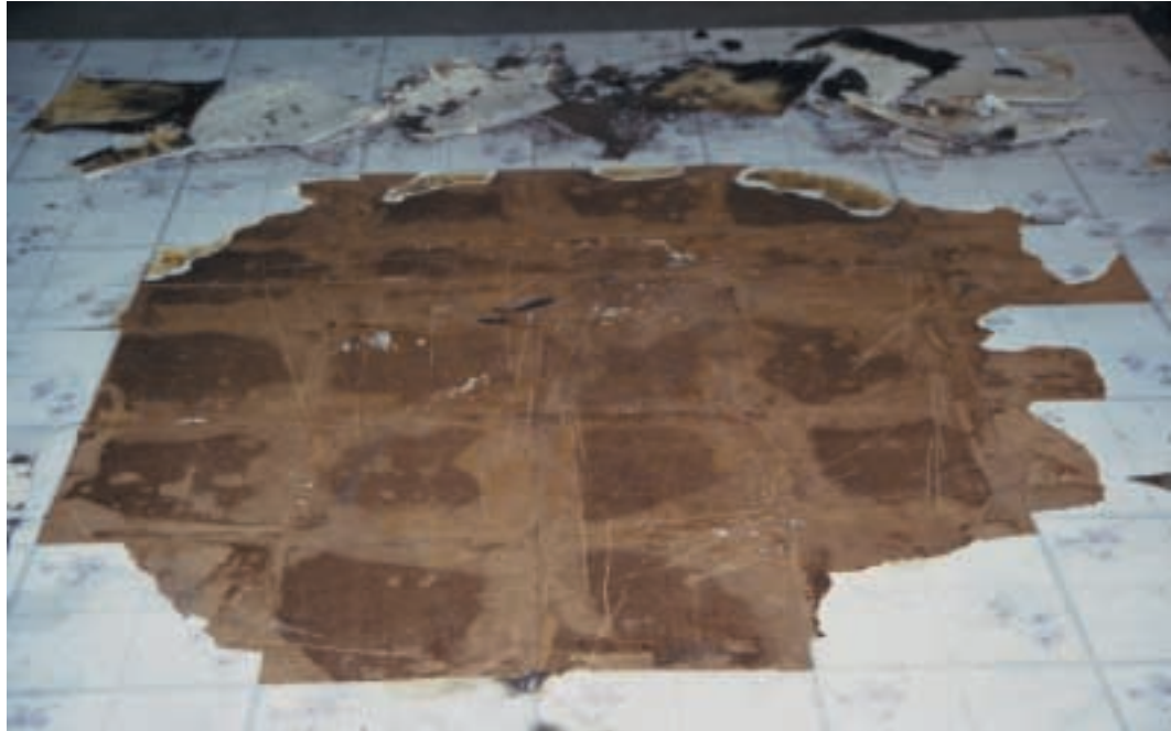
Figure 13. Vinyl tile removed after a 1,000 mL gasoline spill fire. Damage to the fiberboard is limited to the vinyl tile seam locations.
